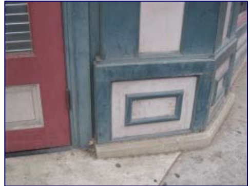
Dirty facade – Building also has dusty grimy windows and chipped siding
