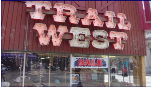
Dilapidated sign band – Posted paper signage – Broken sign
